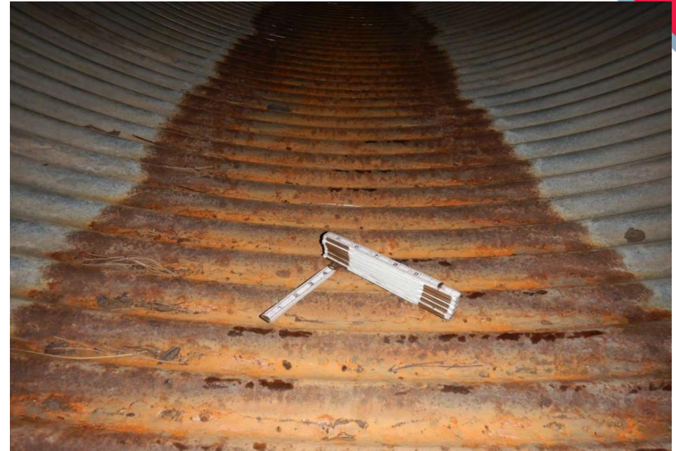
Typical corrosion of pipe invert
