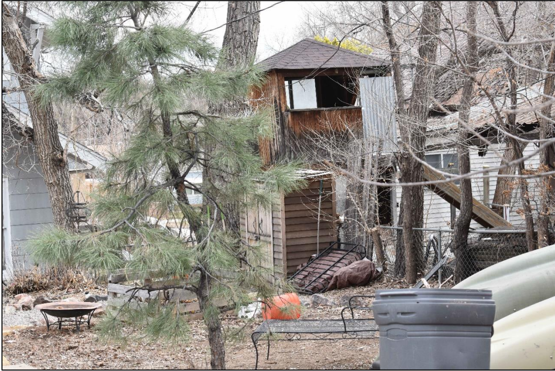
11 of 11. The front and west wall of the small shed on the south property line. View southwest.
