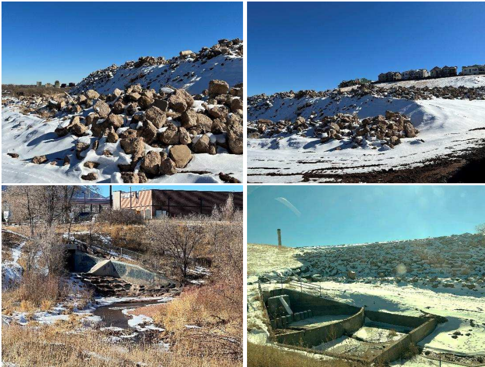
Figure 8. Inadequate Storm Drainage System
