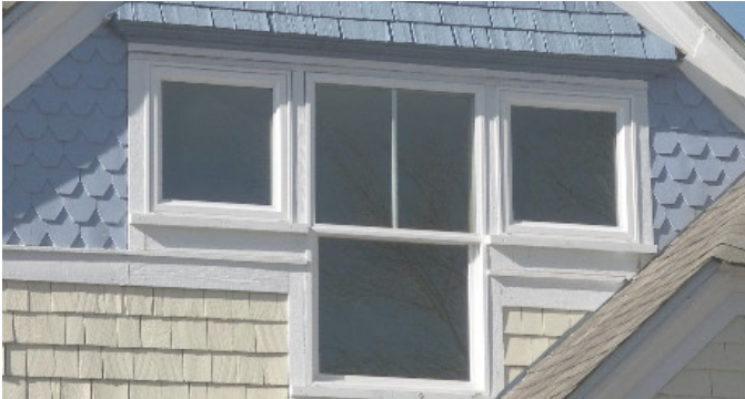
RECOMMEND replacement windows match material, size, jamb profile, and appearance of existing.
