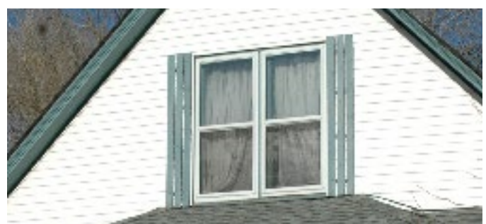
AVOID the addition of shutters which are not of the historical style or appear as false or non-functional.
