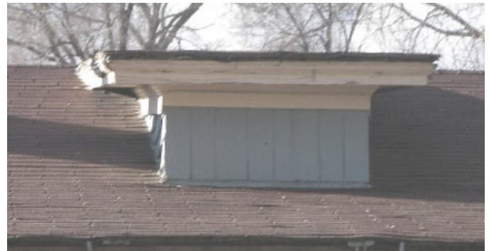
AVOID removing or obscuring original dormer elements and windows.
