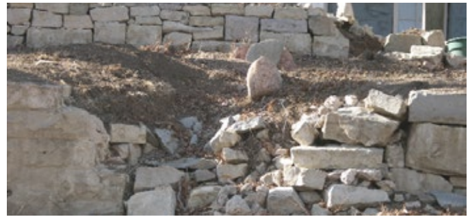
AVOID deferring maintenance on crumbling masonry. Maintain to prevent further deterioration.
