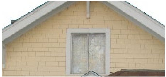
AVOID replacement with aluminum or vinyl windows that do not replicate original unit type.
