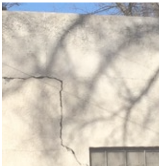
Example of previously painted stucco with cracking deterioration.
