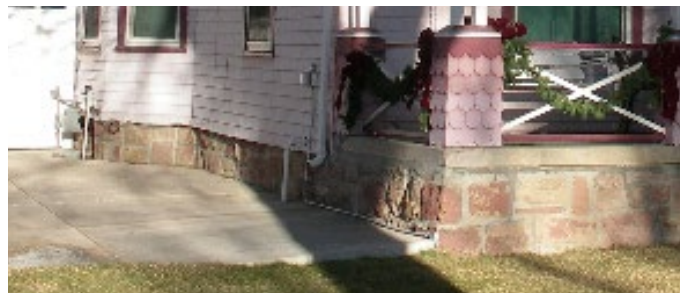
New replacement foundation that uses salvaged foundation stone as a veneer over new poured concrete foundation walls. Height of new foundation preserves the original podium relationship of height of floor above surrounding ground.
