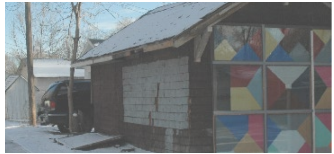
AVOID allowing deteriorated conditions and the use of non-historic replacement materials for outbuildings.
