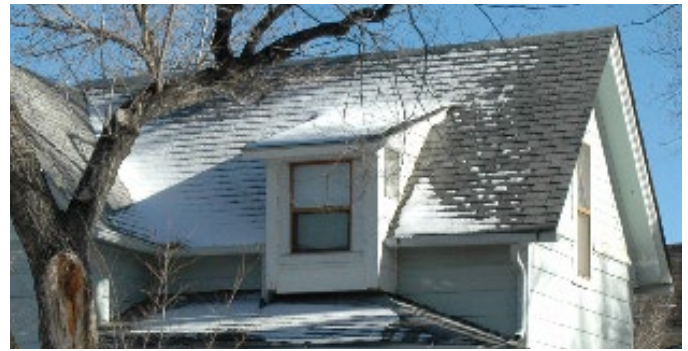
AVOID installing new dormers that do not replicate the existing building roofline.
