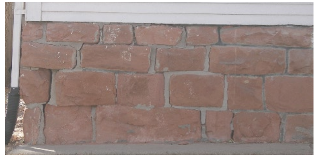
AVOID delaying the repair of obvious foundation deterioration.
