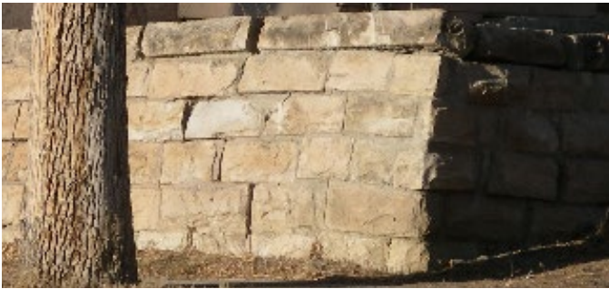
RECOMMEND re-use of historic masonry materials when they can be salvaged and re-applied.
