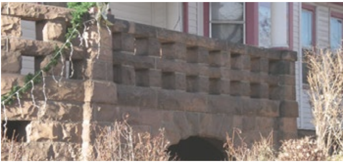
RECOMMEND maintaining existing historic foundations.
