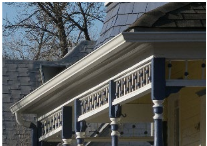
Example of gutters in good condition and connected to downspout to convey water away from building.
