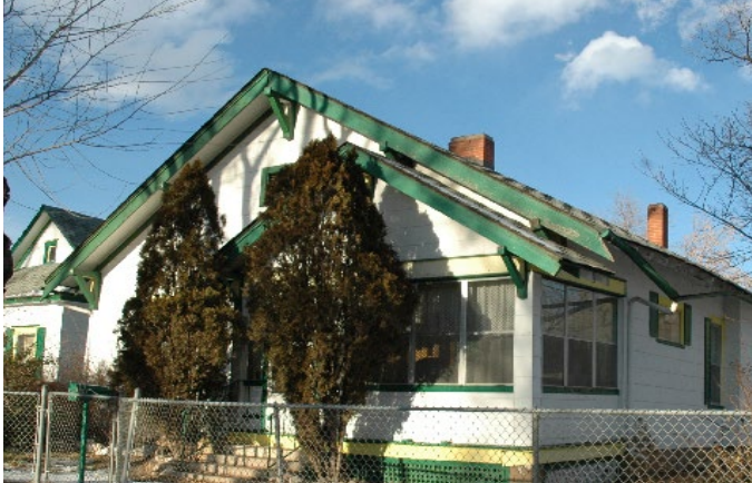
AVOID planting too close to foundations and using oversized shrubs or trees.
