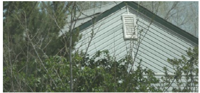
AVOID installation of replacement siding that does not match historic patterns and widths.
