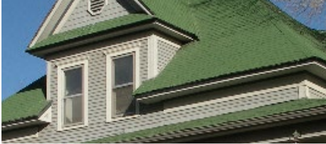
Example of well-maintained siding and trim. Trim occurs at wall corners, intersections of roof overhangs, around vents and around windows.
