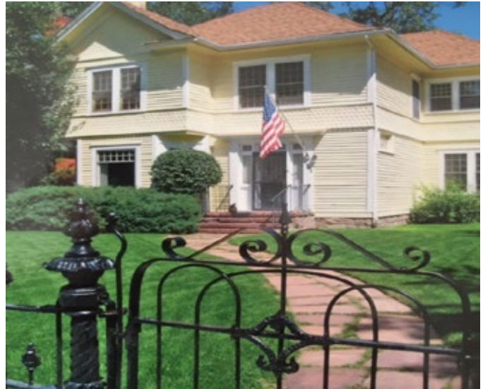
Before: Residence undergoing renovations to replace porch that had been removed and exterior repairs.
