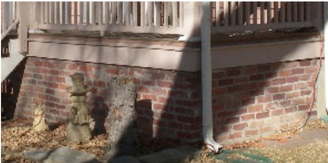
RECOMMEND the salvage and re-use of masonry as a veneer over new foundations. Maintain historic raised foundation relationship above ground.
