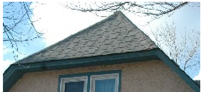
AVOID the use of tee-lock shingles for re-roof projects.
