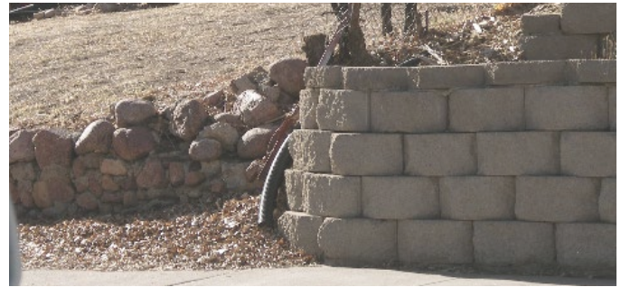
AVOID , wherever possible, replacing salvageable stonework with modern retaining walls.
