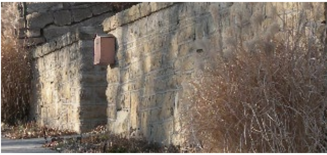
RECOMMEND using correct mortar repairs to match joint softness, joint size, and mortar colors.
