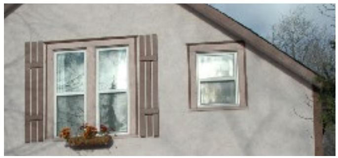
AVOID unpainted bright aluminum finish storm window frame finish.
