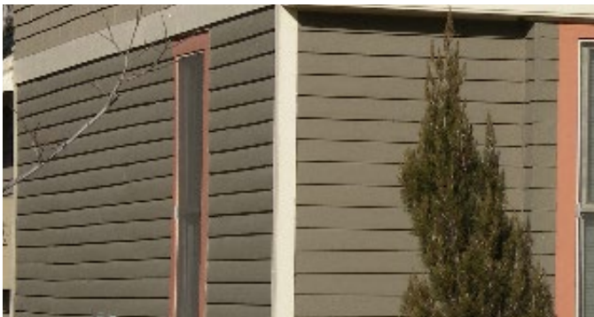
Exterior wall repaired by partial replacement of damaged bevelled cedar siding to match existing siding that has been retained and repaired.
