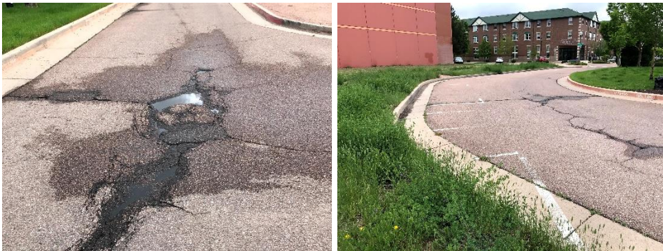
Figure 2. Poor Provision of Street Improvements
