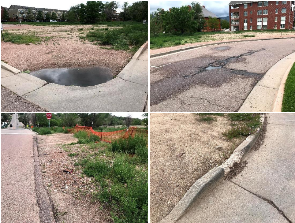
Figure 9. Deteriorated Pavement and Curbs and Missing Sidewalks
