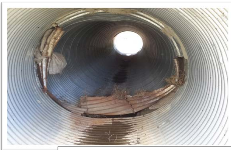
Failing corrugated metal pipe (CMP)
