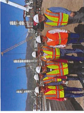
Board Members Murray, Fomune, Donelson, and Avila joined Chief System Planning and Projects Officer, Lisa Barbato, and General Manager of Planning and Design, Joe Awad, to tour Marm Drain Power Plant and see the progress of our natural gas generators in May 2022.
