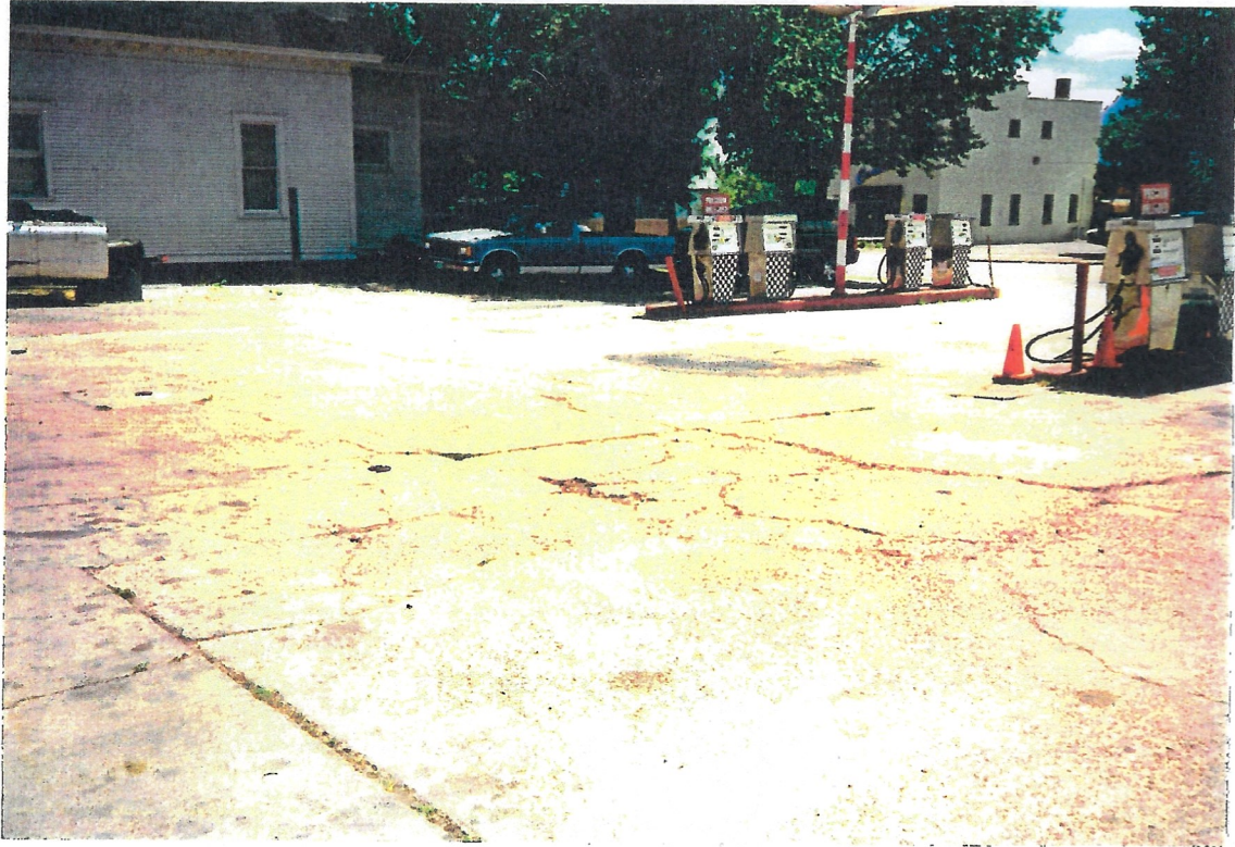
View of parking area and location of the three 8,000 USTs, (left to center of photo)
