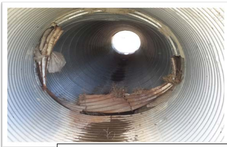
Failing corrugated metal pipe (CMP)
