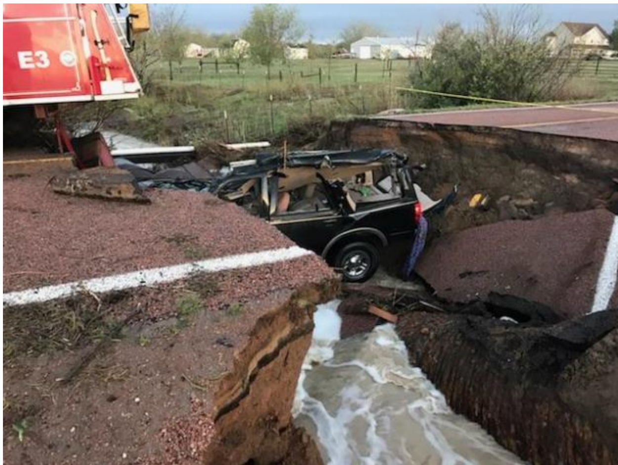
Figure 4-47: Old Pueblo Road After a Sinkhole Trapped Two Cars and a Firetruck on July 24, 2018
