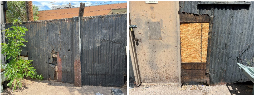
Figure 12. Deteriorated Fences and Walls
