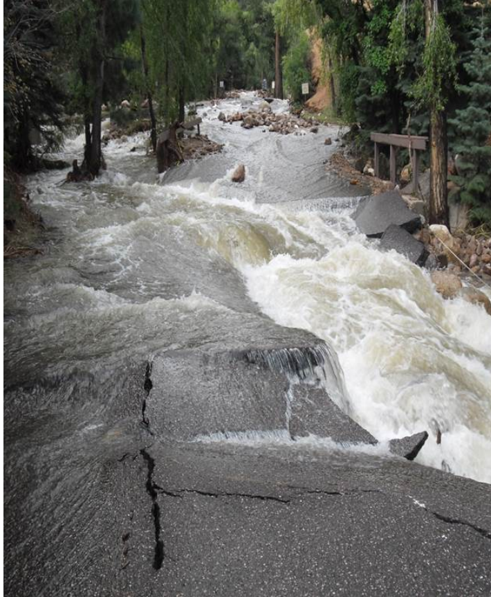
Figure 11. Flooding destroys roadway infrastructure along Cheyenne Creek.
