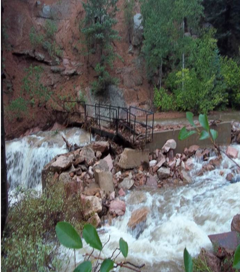
Figure 9. Flood damage to Colorado Springs Utilities water supply infrastructure on Cheyenne Creek.
