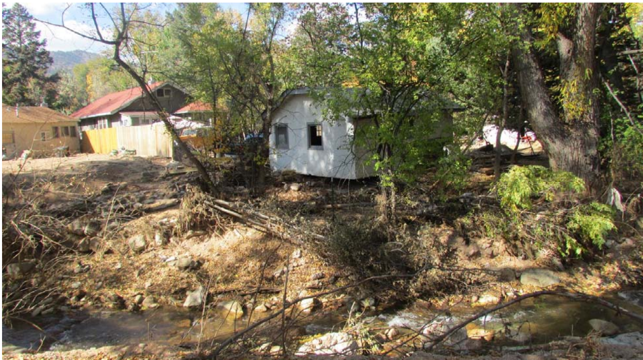
Figure 10. Flood damage to structures on Cheyenne Creek.
