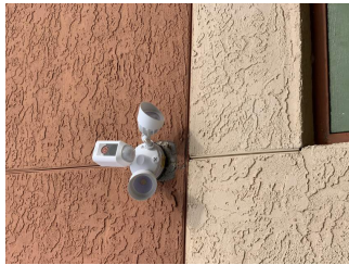
L-1 = Existing Shielded Wall downlight
