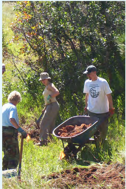
Volunteers lead by a trained crew participate in trail repair. Source: City of Colorado Springs
