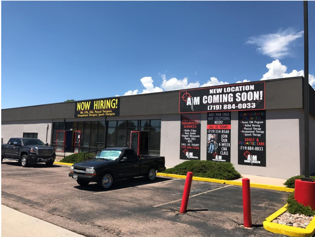
Banner Violations north and west elevations
