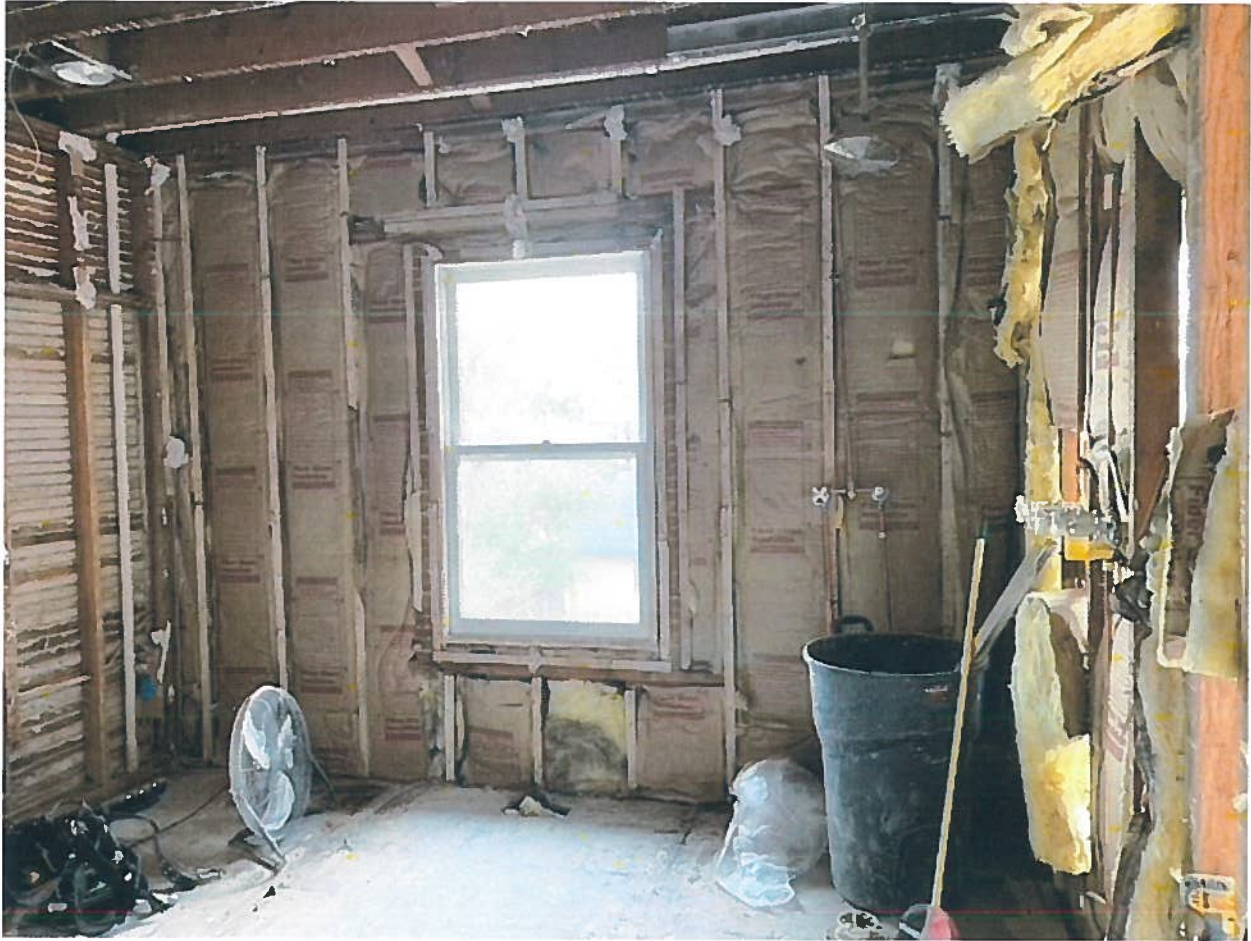
Current view from inside master bathroom. This window does not meet new construction window guidelines as referenced in the appeal and poses a safety threat and privacy issues.
