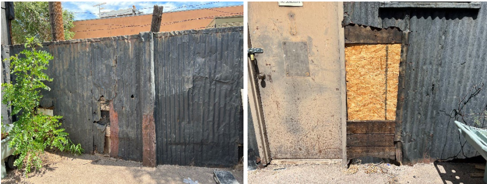
Figure 12. Deteriorated Fences and Walls
