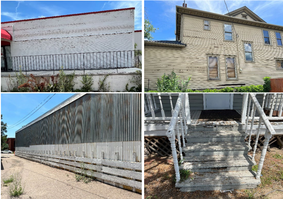
Figure 2. Deteriorated Exterior Finishes and Stairways
