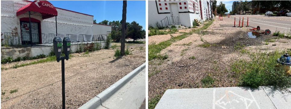
Figure 13. Lack of Sidewalks and Curb
