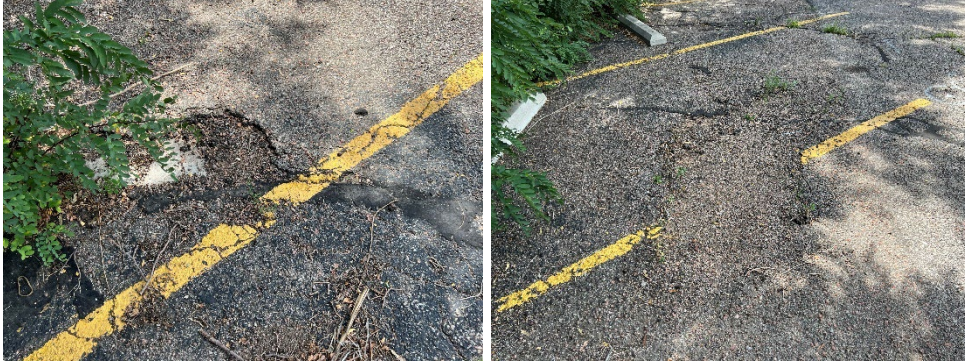
Figure 10. Deteriorated On-Site Parking Surfaces
