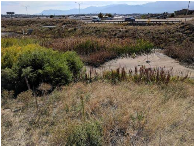
Detention Basin Channel
