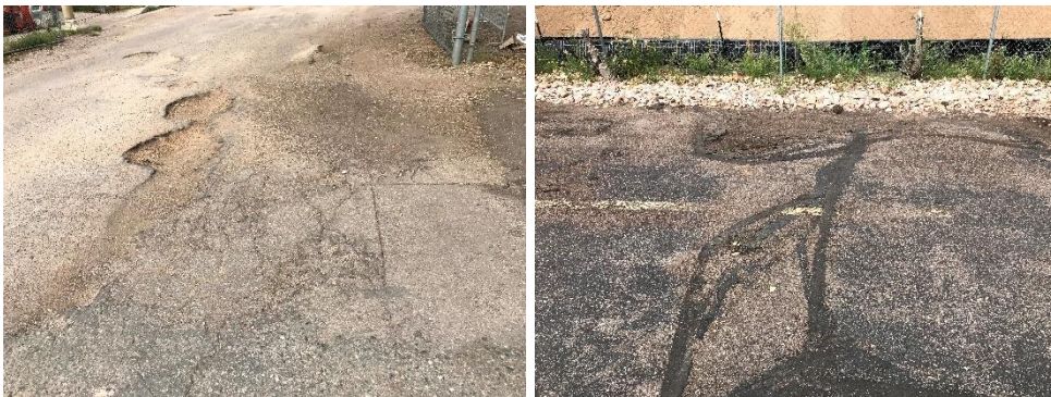
Figure 10. Deteriorated Pavement, Curb, and Sidewalks
