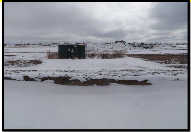
Electrical transformer at Dublin Blvd.
