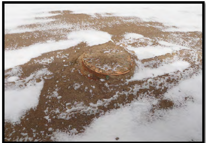
Sanitary sewer manhole in Dublin Blvd.
