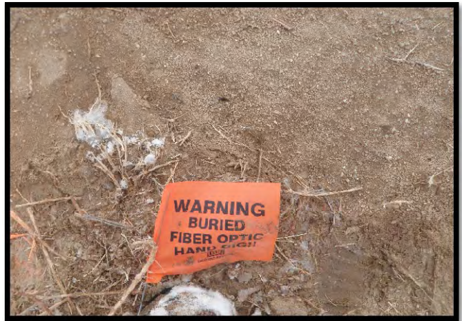
Evidence of fiber optic line in Dublin Blvd.
