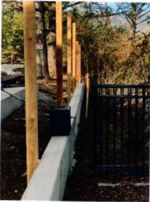
Retaining Wall and filler dirt added in October 2018, six months after driveway. No engineer report stating retaining wall was needed for stabilization prior to October 2018.
