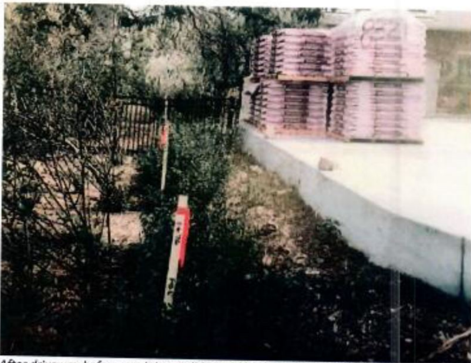
After driveway before retaining wall (taken by Creative Outdoor Living Stakes represent property line inches from where retaining wall was erected.
