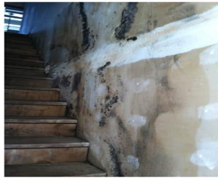
Mold damage in marijuana grow house
