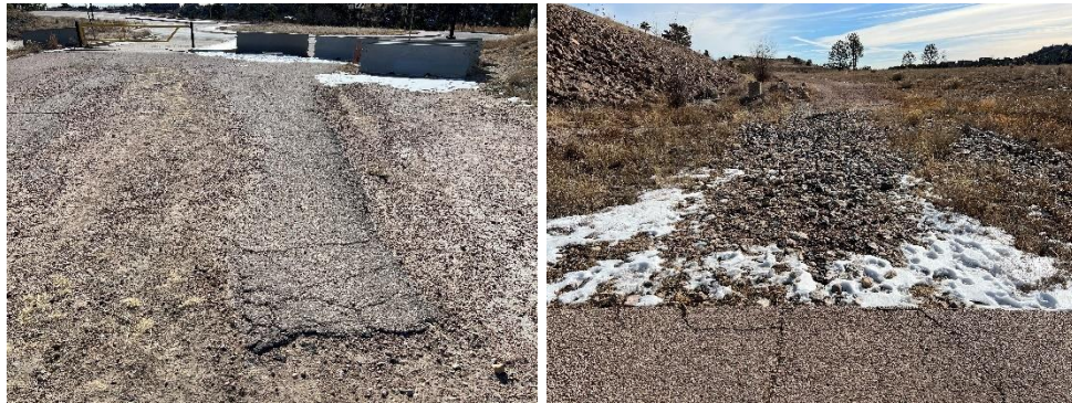
Figure 3. Poor Provision of Street Improvements for Vehicular Traffic
