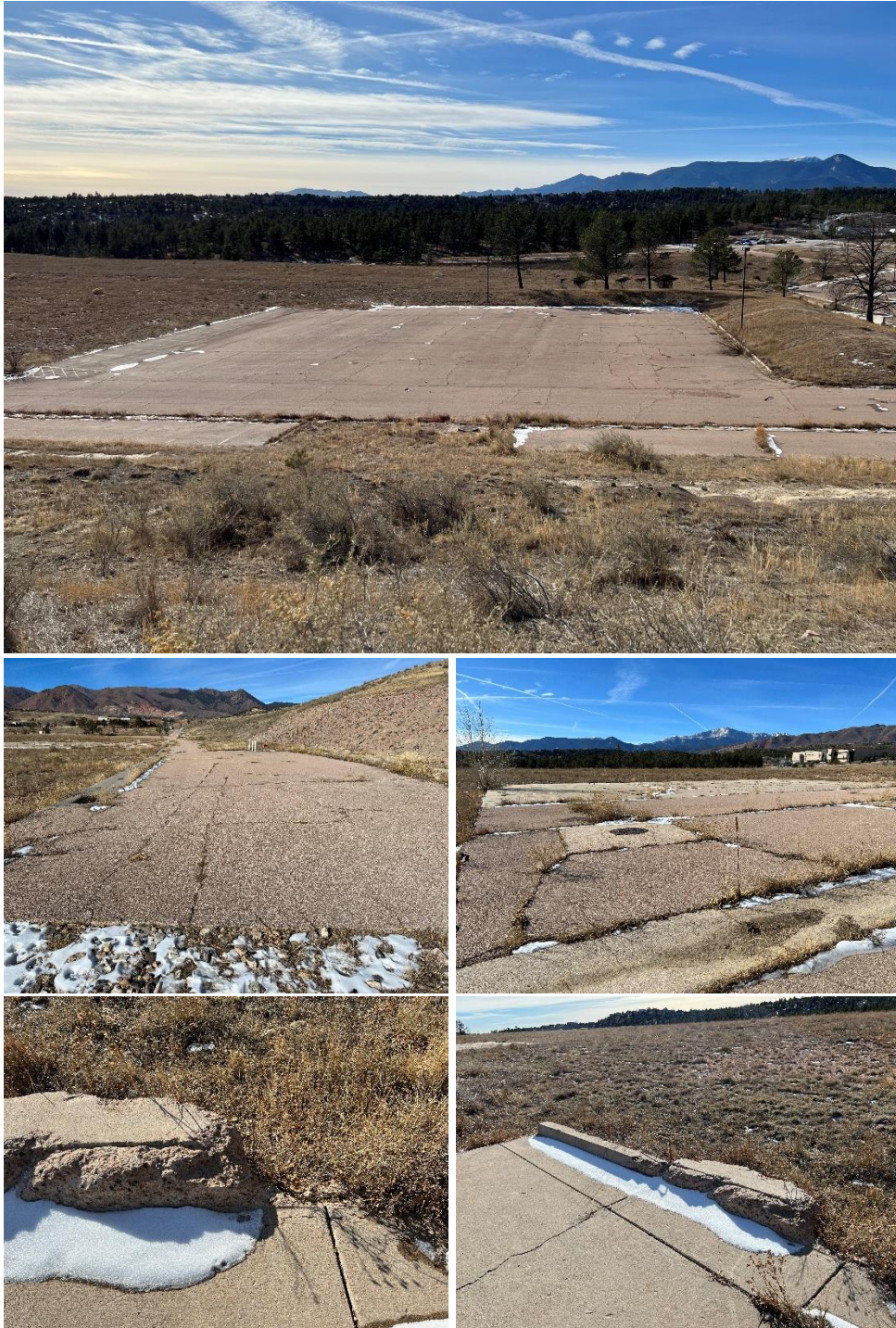
Figure 8. Deteriorated On-site Parking Surfaces and Curbs
