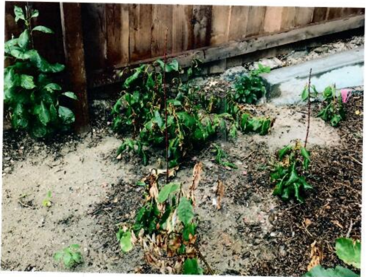
Photo D: Runoff at End of Retaining Wall
