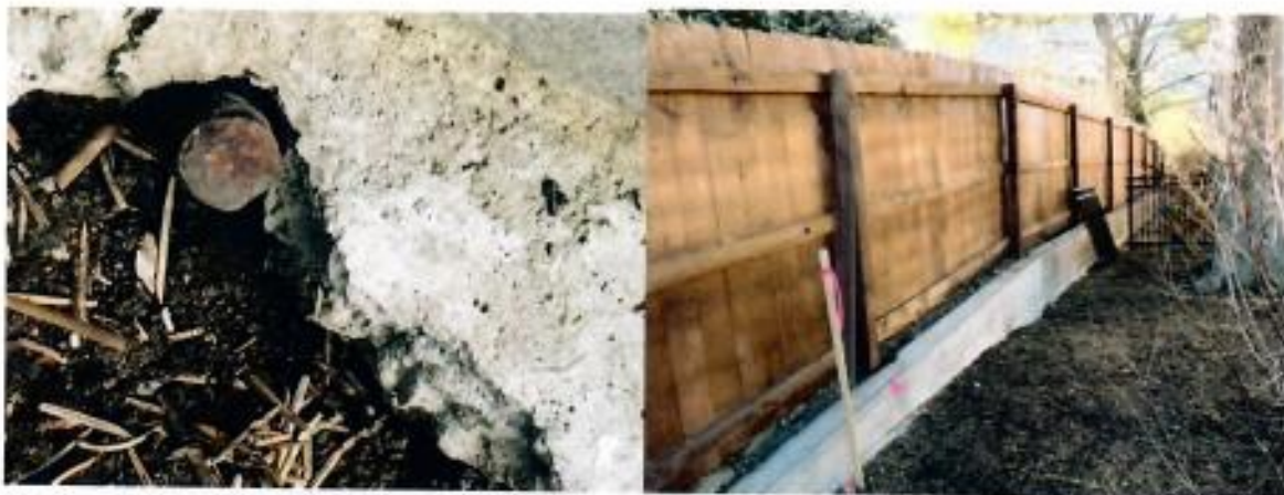
Retaining wall falling apart is inches from property line
