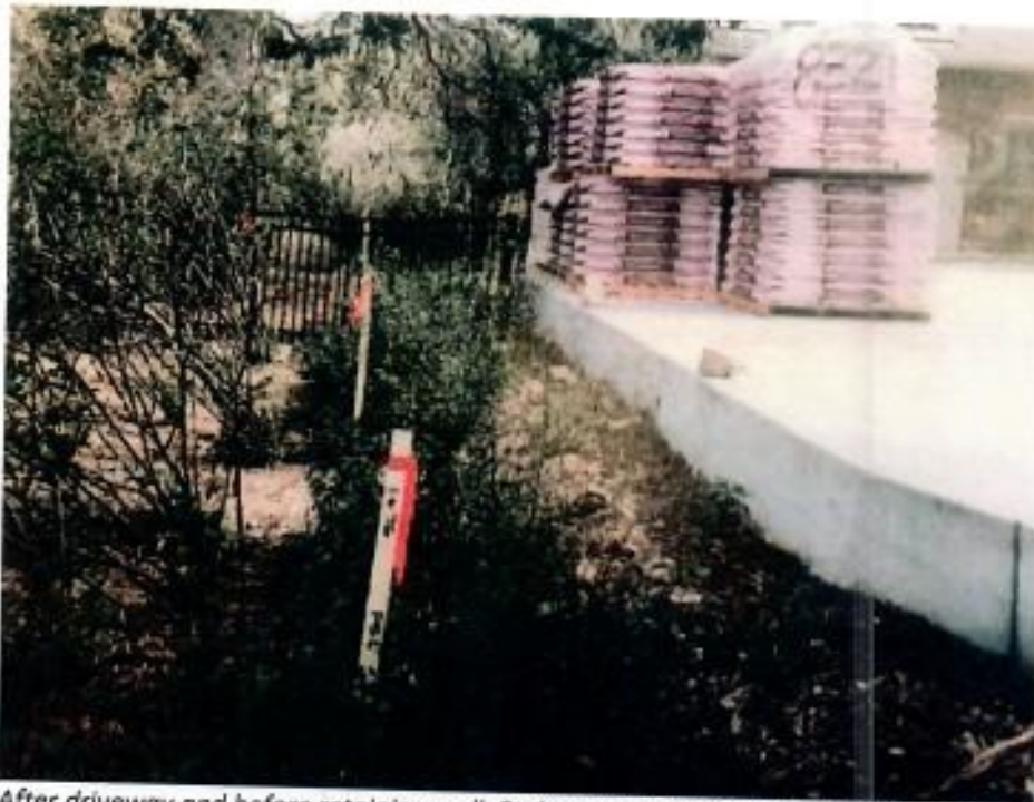
After driveway and before retaining wall. Stakes represent property line inches from where retaining wall was erected.
