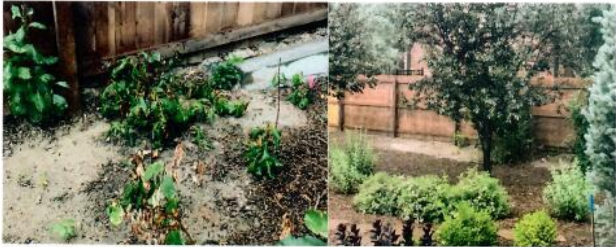
Ongoing damage to appellants' property caused by stormwater runoff
