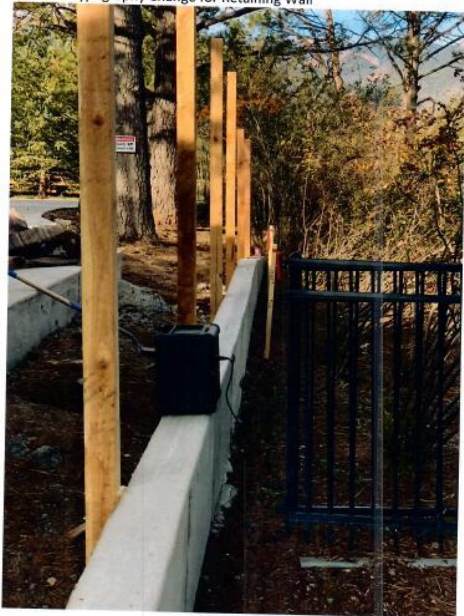
Photo B: Typography Change for Retaining Wall
