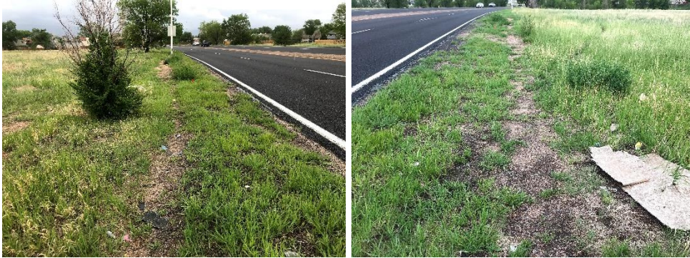
Figure 2. Lack of Sidewalks
