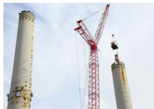
A crane systematically demolishing one of the stacks at the Drake Power Plant
