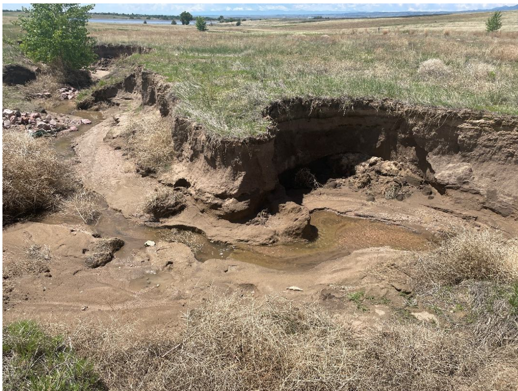
Figure 7 (Station 4+50): Bank failure within reach (looking downstream)
