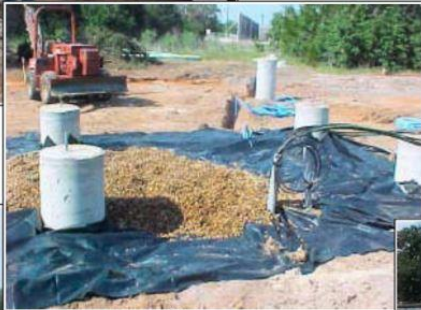
Underground Electrical, Phone and Signal
