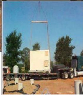
Ground System includes 1200' of 4/0 Copper cable, 12 ground rods, exothermic connections tested to FAA specifications.
