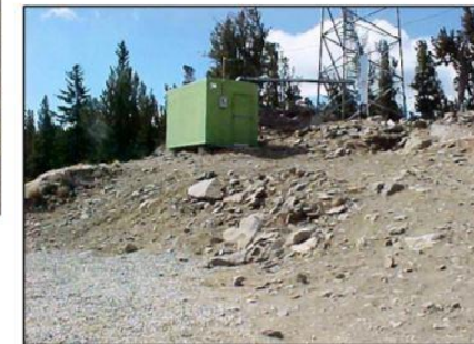
Move this shelter to new location, install customer's equipment for temporary service.
