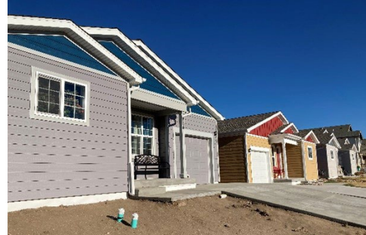
New Habitat for Humanity home under construction Photo credit: KRDO Grocery Services
