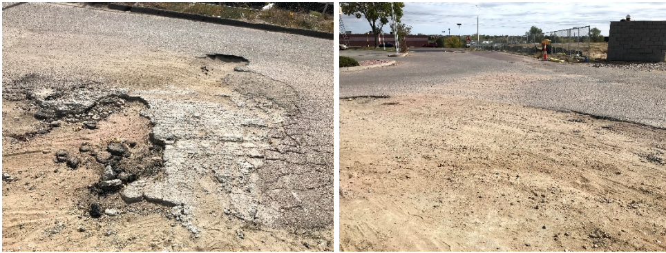
Figure 2. Poor Provision of Street Improvements
