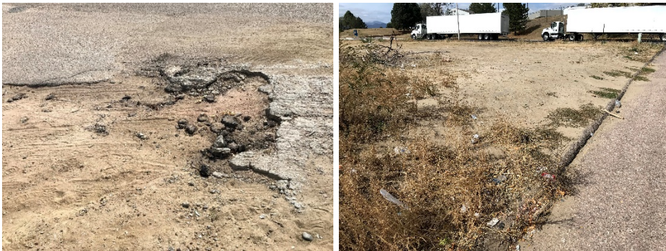
Figure 10. Deteriorated Pavement and Curbs and Missing Sidewalks
