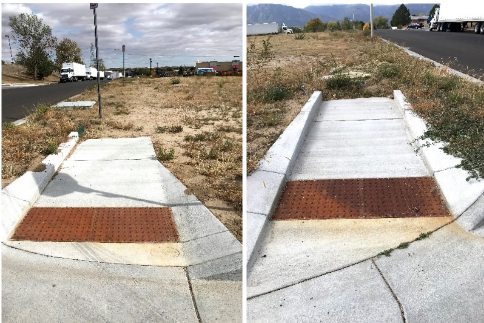
Figure 3. Lack of Sidewalks
