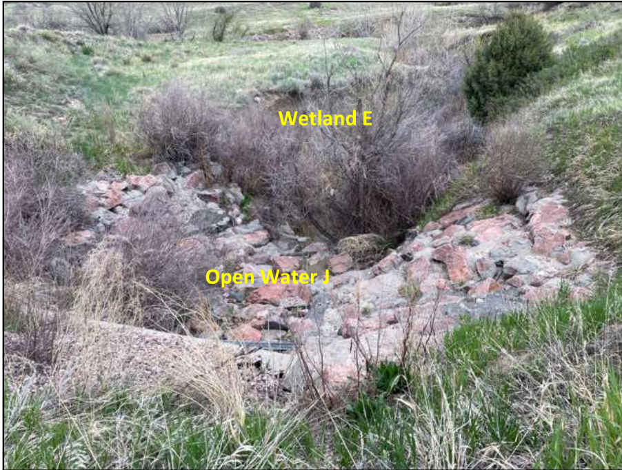
9. Photo taken from path on top of a 48-inch diameter culvert and facing east/downstream. The Wetland E channel is deeply incised, but vegetation is well-established. Open Water J consists of grouted riprap at the culvert outflow, flows were a trickle and below the ordinary high water mark. May 21, 2021.
