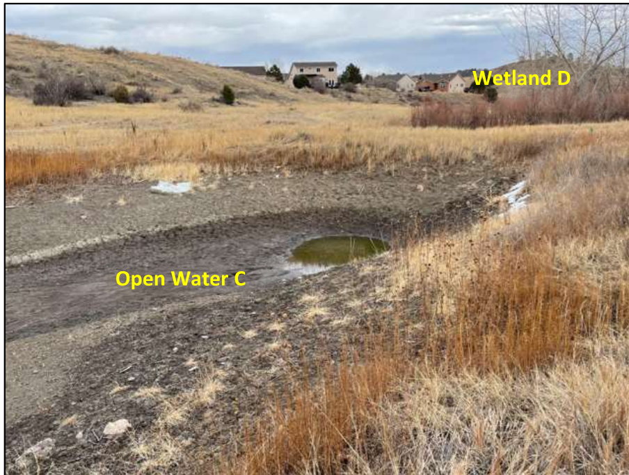
5. Photo facing northeast across Open Water C (pond) when it was almost dry. The pond is formed by an access road that functions as a dam. There is no culvert to convey surface flows downstream of the pond. March 8, 2021.
