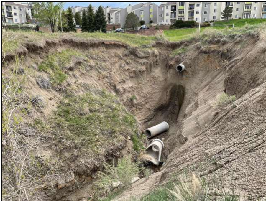
10. Stormwater outlet at the top of the eroded gully (Open Water F). Photo is facing south toward S. Rockrimmon Boulevard. Runoff appears to come from roads and a detention basin in the apartment complex. May 21, 2021.
