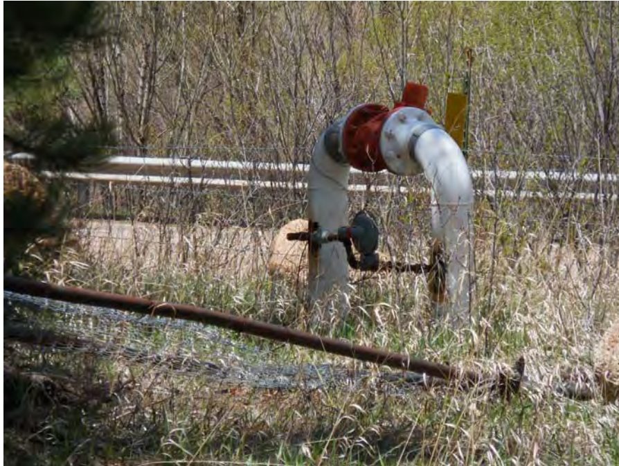
Utility infrastructure shown in prior photograph looking north with Highway 24 in background.
