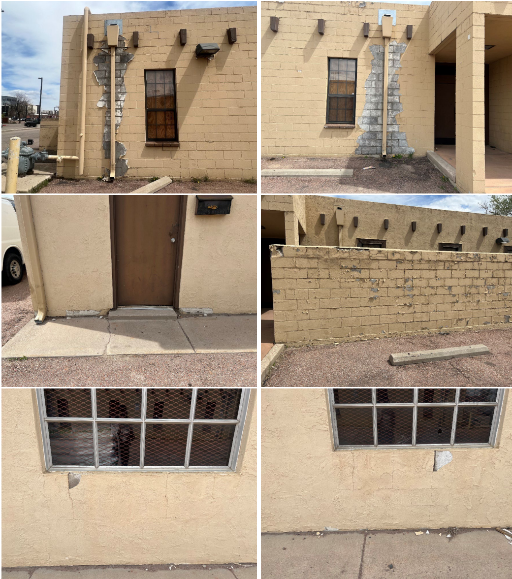
Figure 2. Deteriorated Exterior Finishes
