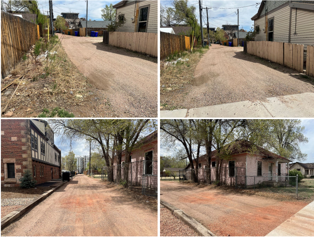
Figure 12. Lack of Pavement
