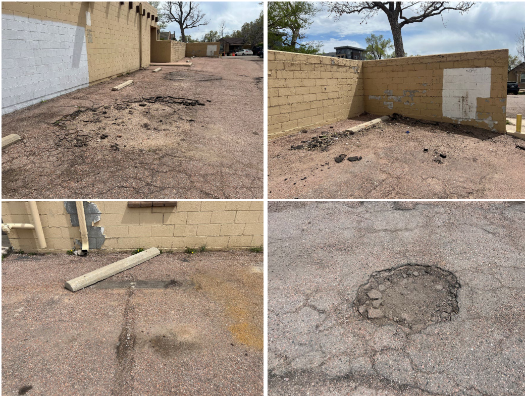
Figure 9. Deteriorated On-site Parking Surfaces
