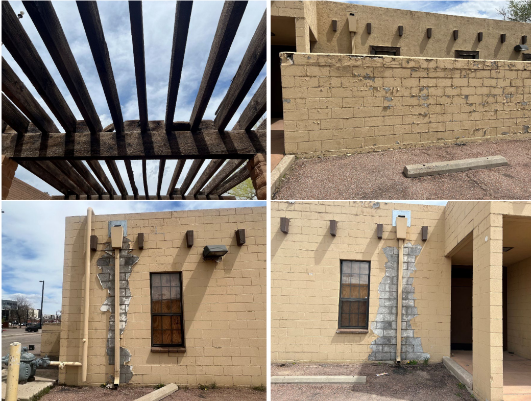
Figure 8. Deteriorated Walls and Pergola
