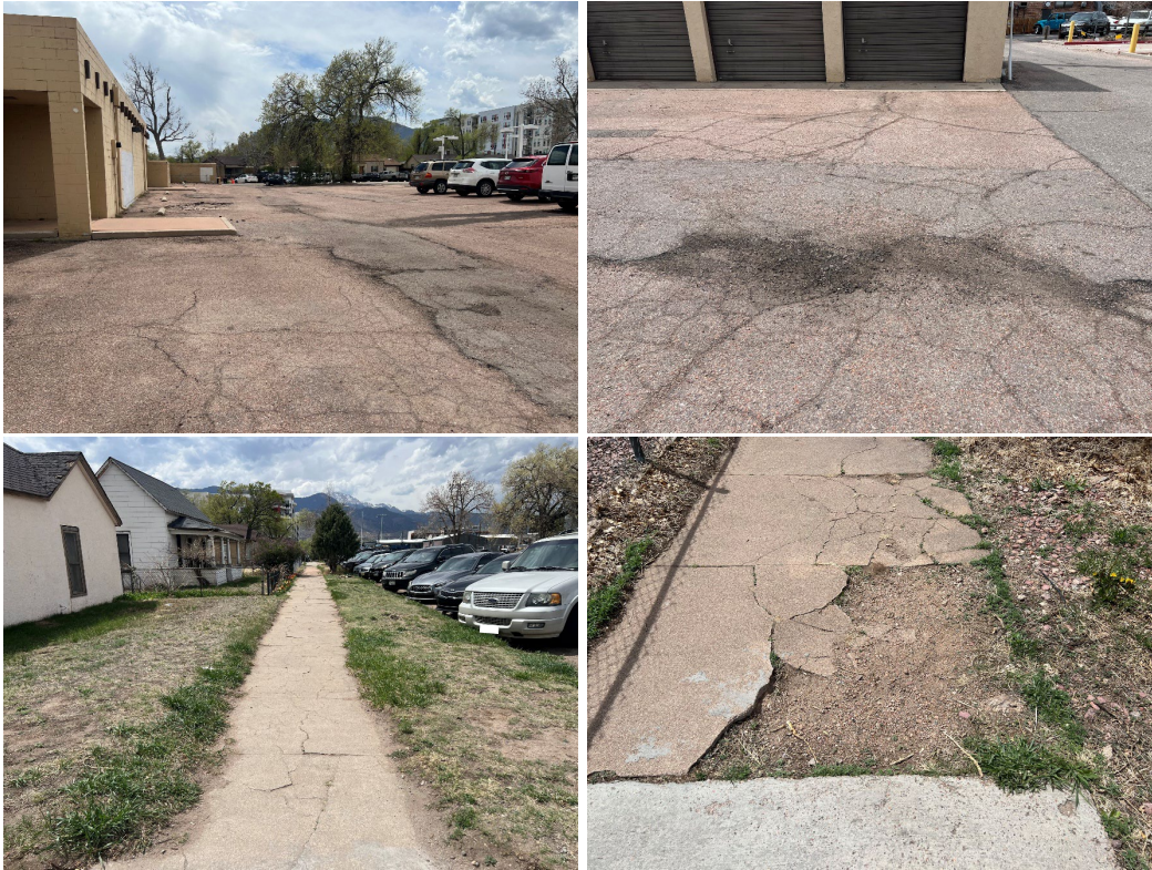
Figure 11. Deteriorated Pavement and Sidewalks
