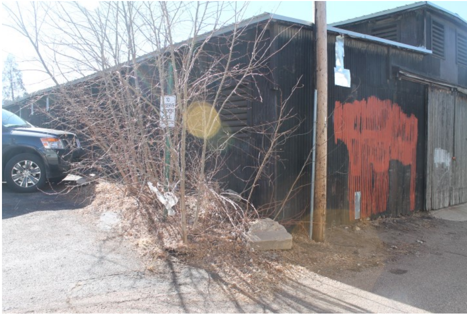
Figure 2-12 Deteriorated exterior walls, deteriorated fascia/eaves, lack of gutters/downspouts, vagrants/graffiti/vandalism, inadequate site maintenance, non-conformance to site development regulations (Photo E-1)
