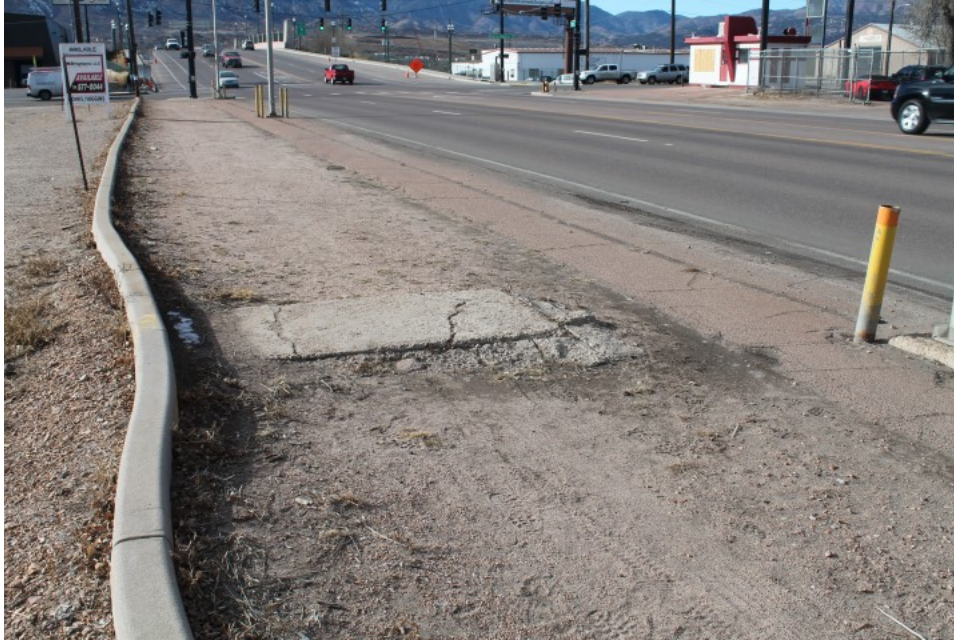
Figure 2-2 Substandard driveway/curb cuts, cracked or uneven pedestrian surfaces, unsafe level changes, deteriorated curb and gutter, inadequate and deteriorated sidewalk, non-conformance to development regulations (Photo A-3)
