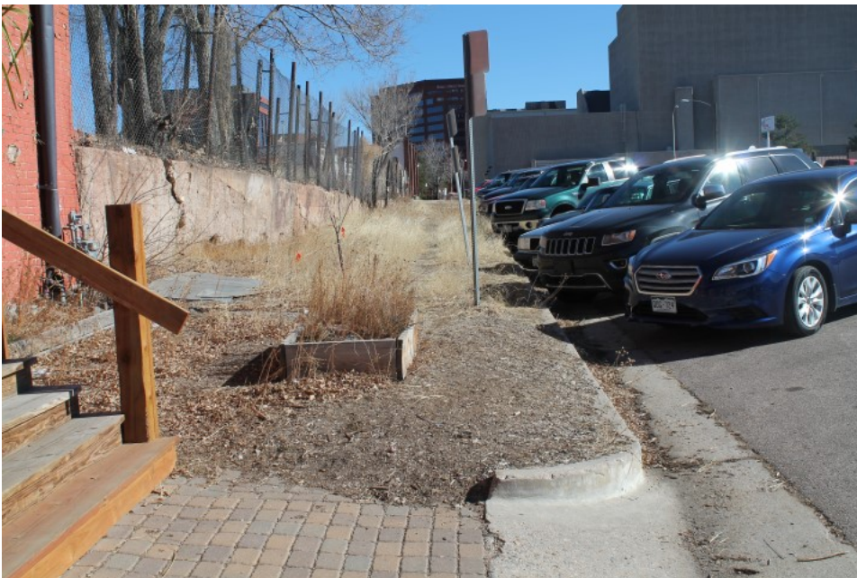
Figure 2-11 Poor vehicle access, substandard driveway/curb cuts, cracked or uneven pedestrian surfaces, unsafe level changes, inadequate and deteriorated sidewalk, presence of trash and debris, unsafe level changes, inadequate site maintenance, non-conformance to development regulations, deteriorated site walls (Photo D-10)
