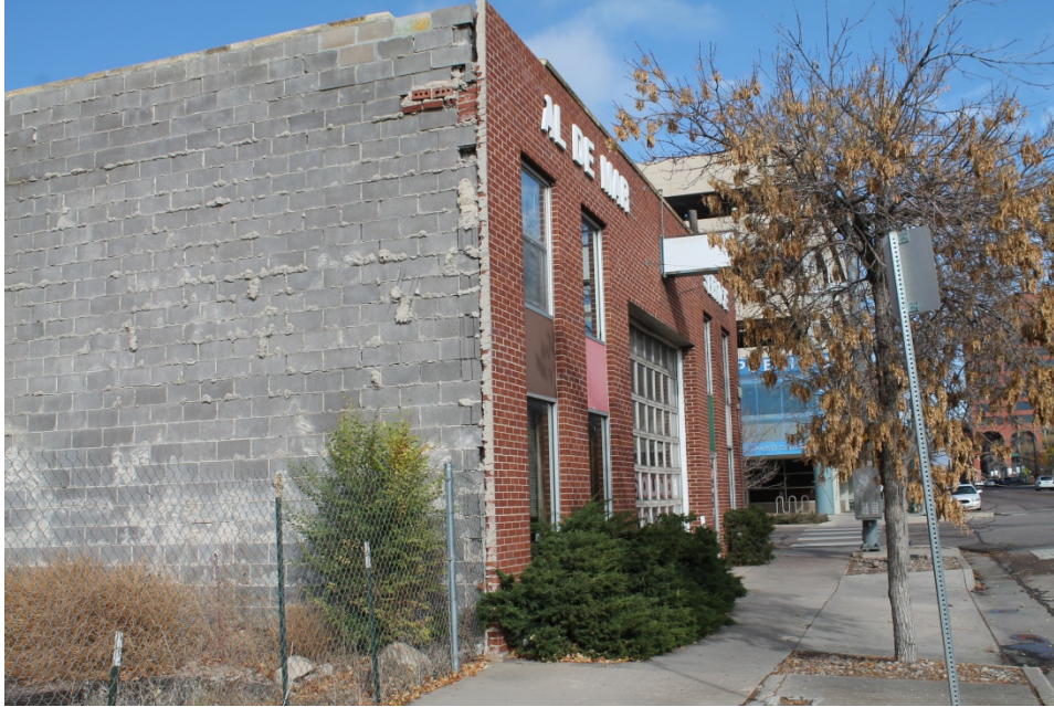
Figure 2-3 Deteriorated exterior walls; deteriorated exterior finishes; deteriorated doors and windows; cracked or uneven pedestrian surfaces; presence of trash and debris; potentially hazardous materials and conditions; deterioration of signage; trees and shrubs in high traffic areas (Photo 5)
