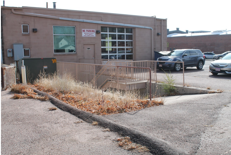
Figure 2-5 Deteriorated loading areas/ramps; cracked or uneven pedestrian surfaces; poor drainage; presence of trash and debris; potentially hazardous conditions; unsafe level changes; deteriorated parking lot pavement; lack of sidewalks or pedestrian areas; deteriorated surface drainage; inadequate site maintenance; lack of conformance to site development regulations; dry debris near structures; unsafe level changes (Photo 9)
