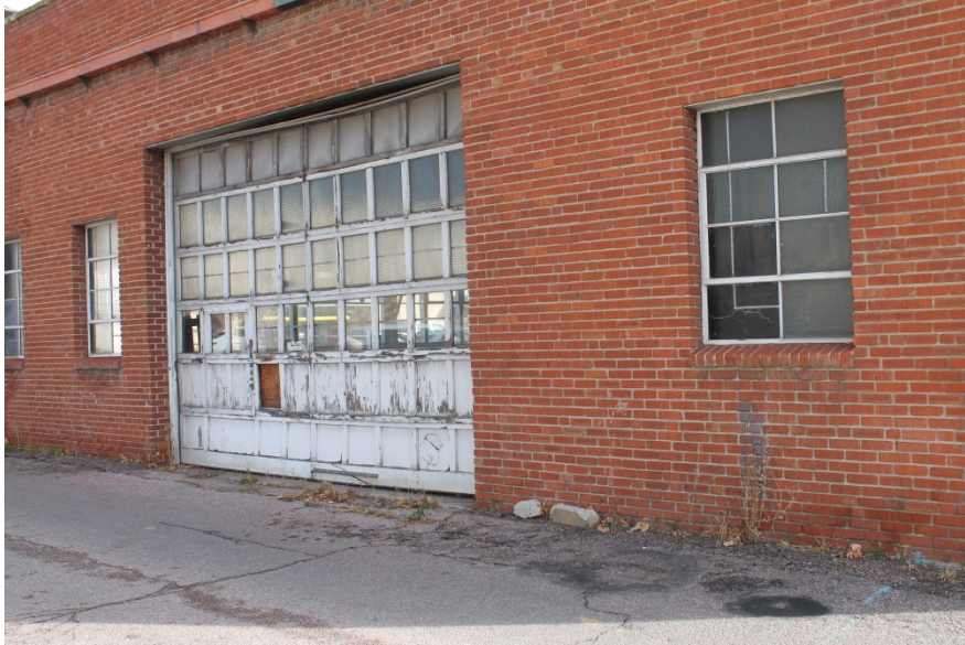
Figure 2-1 Deteriorated exterior walls and finishes; deteriorated windows and doors; deteriorated loading areas; presence of debris adjacent to structure; debris near high traffic areas; Inadequate site maintenance; non-conformance to development regulations; presence of debris next to structures (Photo 1)
