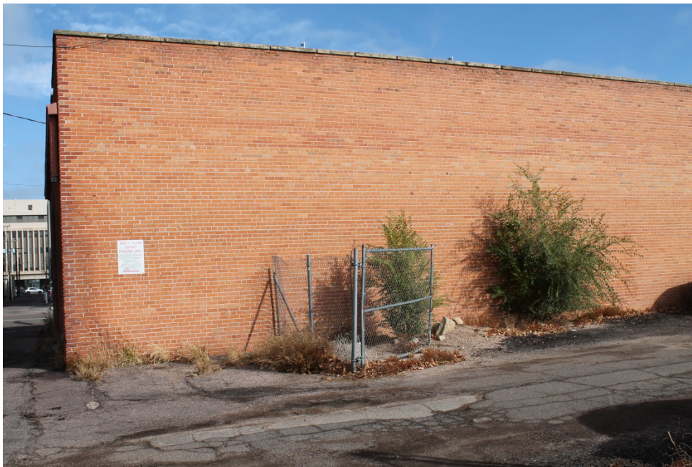
Figure 2-6 Deteriorated external walls; deteriorated exterior finishes; deteriorated gutters/downspouts; deteriorated walls/fences/gates; cracked or uneven pedestrian surfaces; presence of trash and debris; deteriorated parking lot paving; inadequate site maintenance, non-conformance to development regulations (Photo 12)
